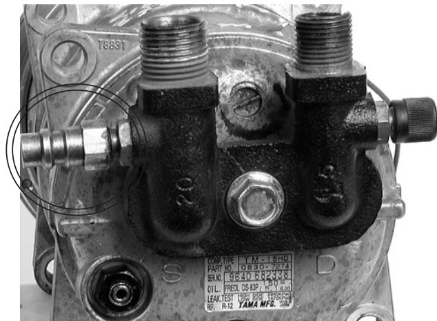
Retro-fitted to 134a, system not flushed.
