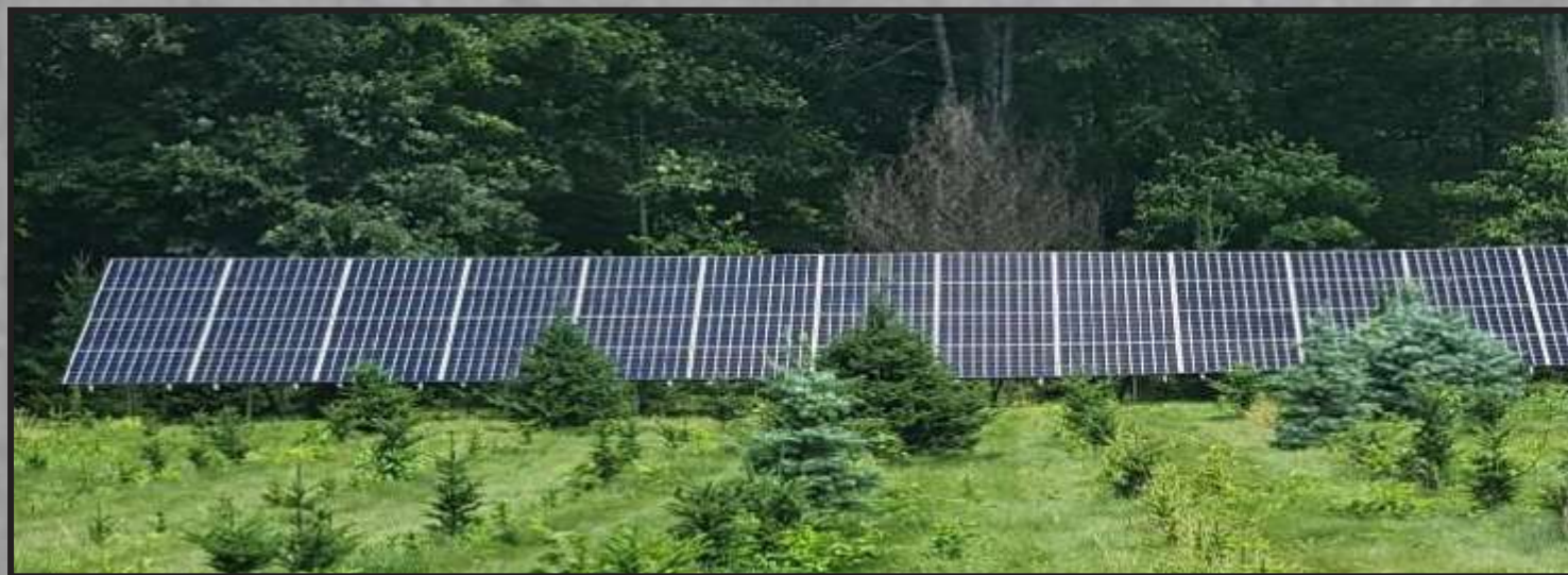
With the help of the USDA, RI DEM, NATIONAL GRID, FARM CREDIT EAST, and others we installed a ground mounted Solar Array 18.56kW(AC) System that was turned on October, 2018.
